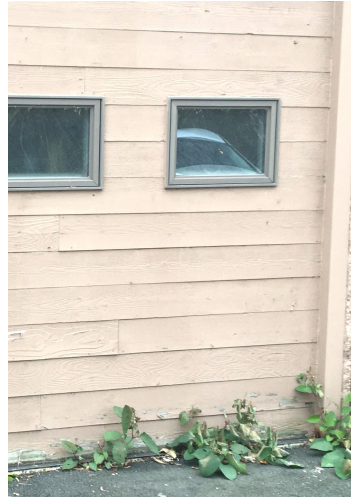
Building envelope has significant water and vegetation intrusion. Several exterior doors were not weather-proofed properly and require complete refinishing or replacement
