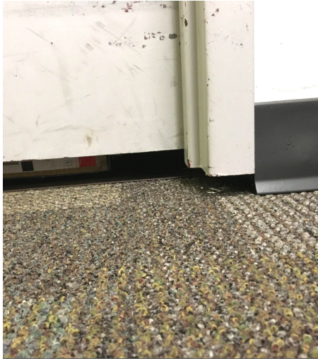
Floors are sinking into improperly created fill, slowly detaching from walls of the building
