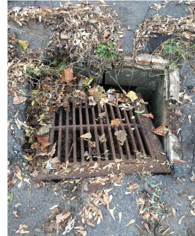
Improper fill is sinking, also causing collapse of drainage systems, potentially compromising environmentally sensitive areas with parking lot runoff as well as being a safety and liability hazard
